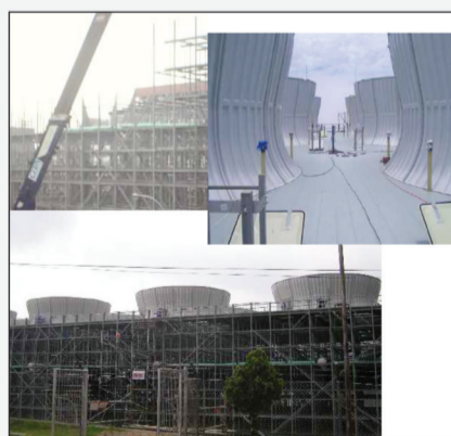
Wayang Windu Geothermal #2 project 2008 (FRP Tower)
